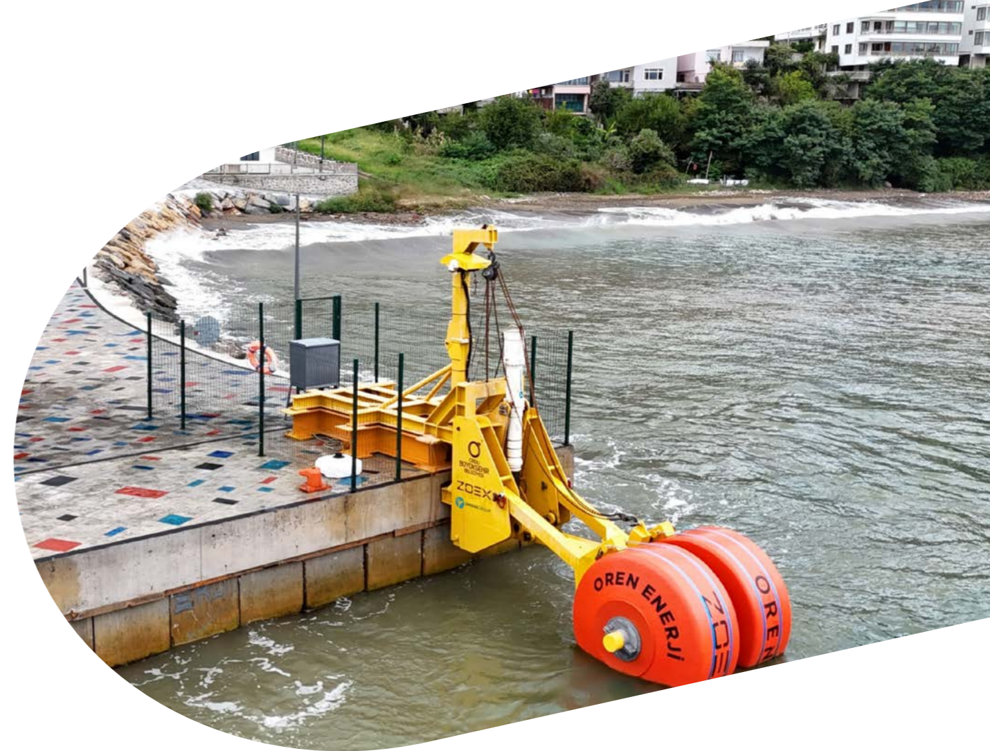
▲ The UMBRAGROUP Power Take-Off installed on the ZOEX Wave Energy Converter.
